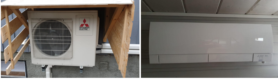
(a) Outside heat pump. There are two of these outside the house. (b) Inside heat pump. There are four of these inside the house.
